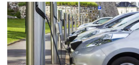
Electric Vehicle Charging Point
